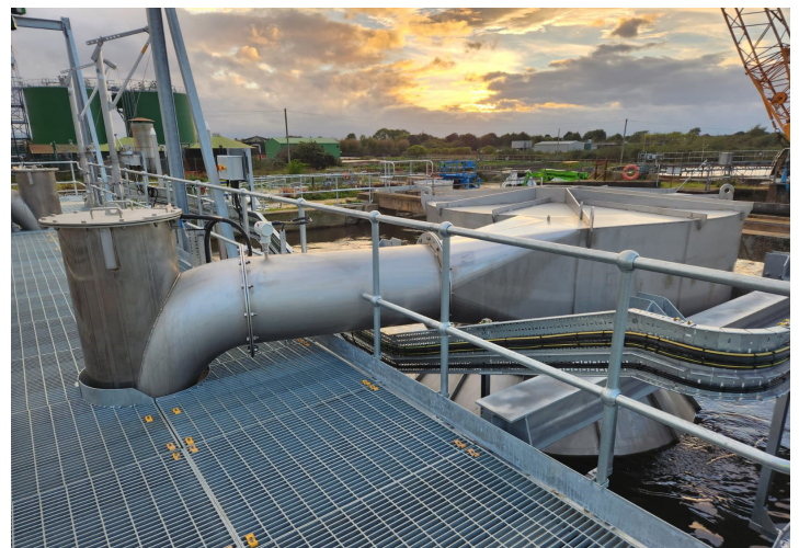
Figure 4. A VPA unit operating in an oxidation ditch
